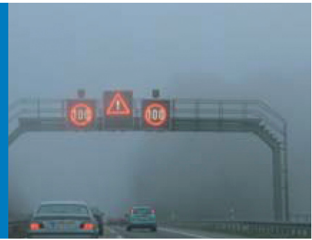
Traffic management systems
